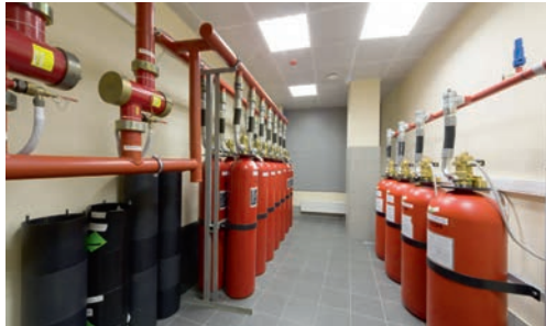
Integrated and intelligent fire systems that sense, detect and prevent is predicted to usher in accelerated growth. (Photo: Pavel Losevsky/Adobe Stock)
